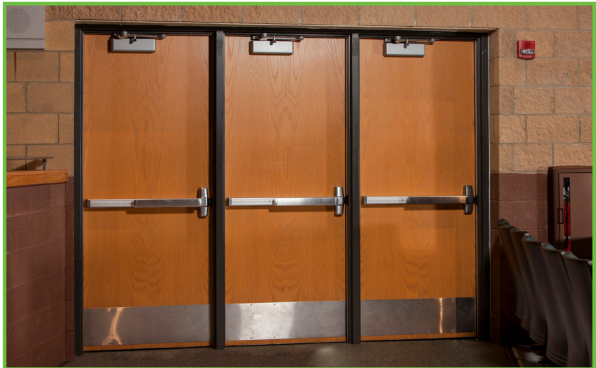
The 2021 I-Codes require hardware operated by a pushing or pulling motion to unlatch with a maximum force of 15 pounds.
